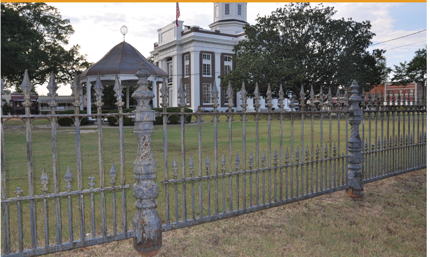
11 | West side of fence: rusted out post bottoms.
