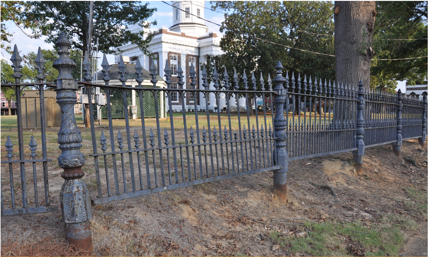
10 | Northeast corner of fence: Broken connection at post.
