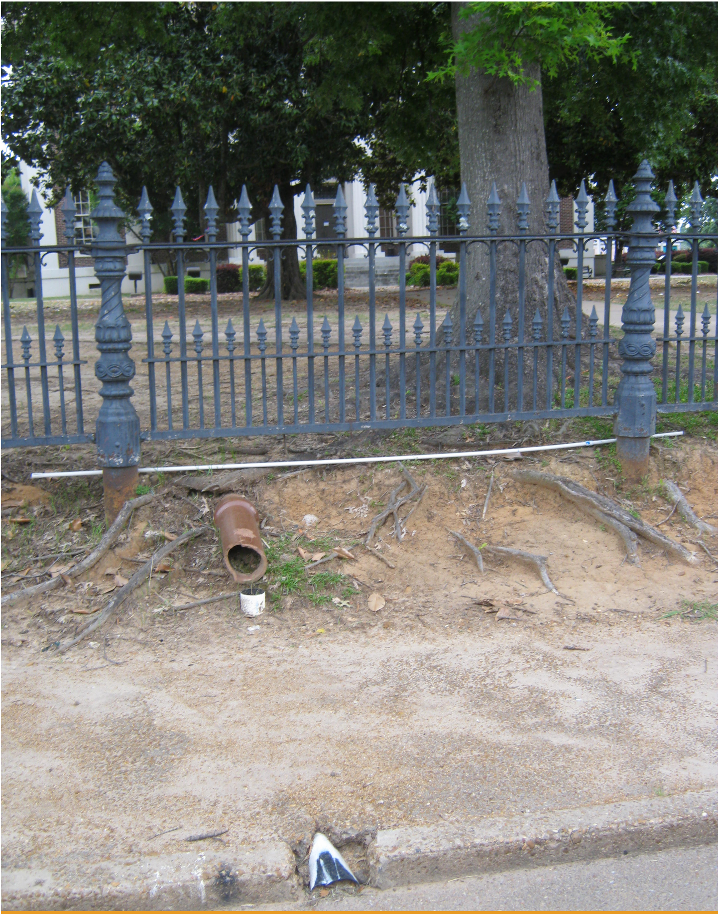
12 | South side of fence: Invasive Tree Roots.
