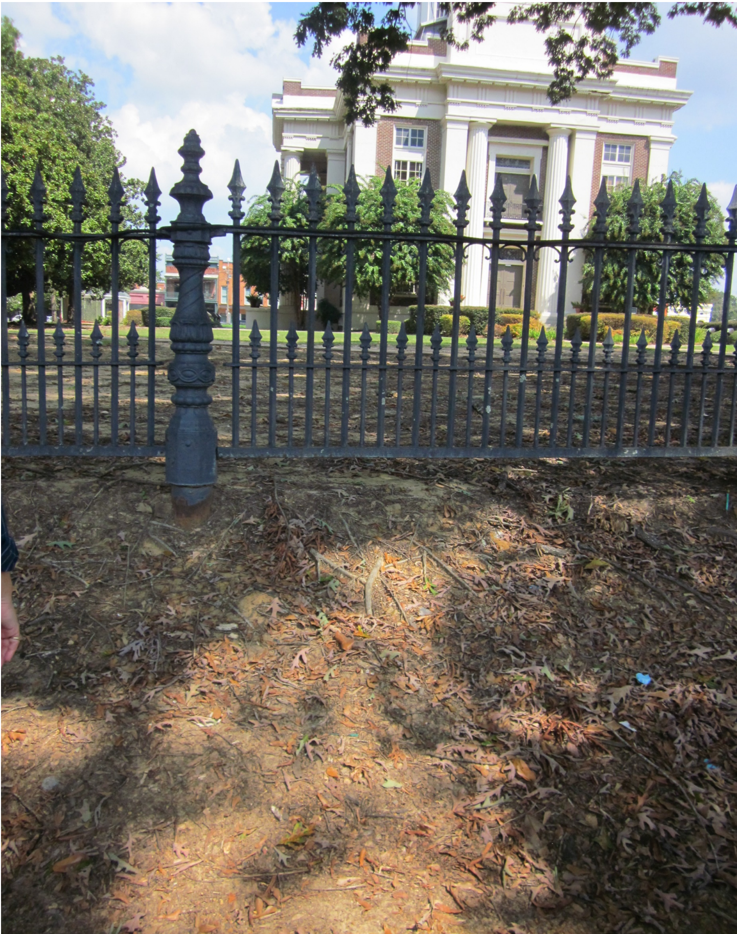
13 | North side of fence: sagging.
