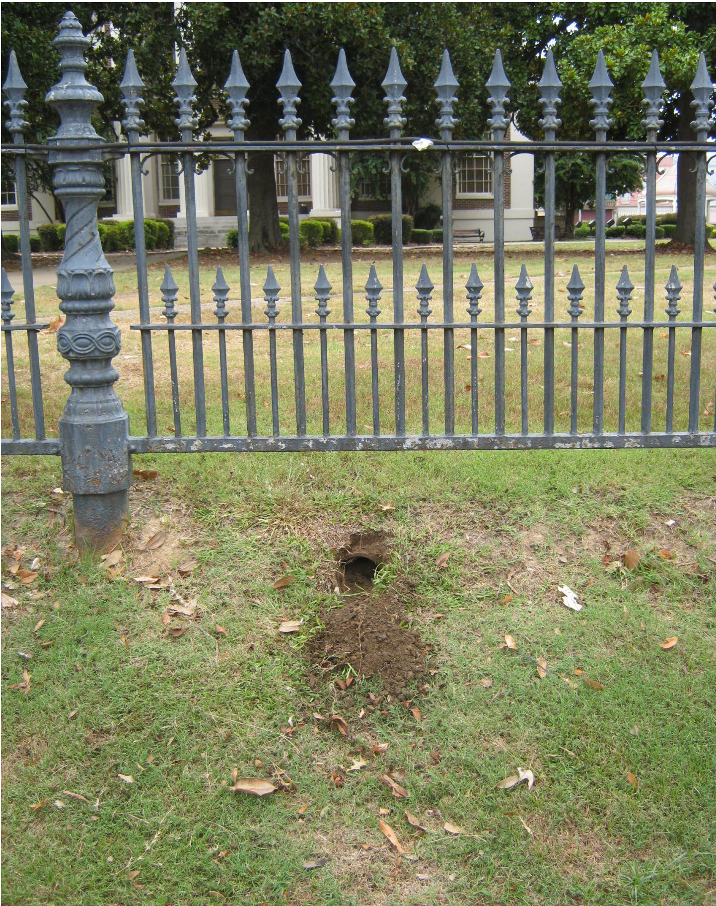
07 | South side of fence: Chipping Paint.
