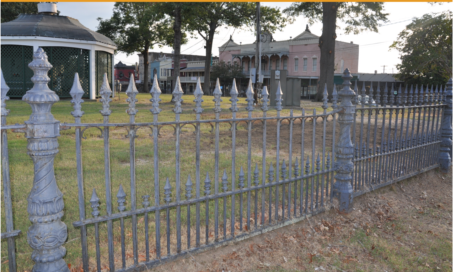
02 | North side of fence: broken finials.
