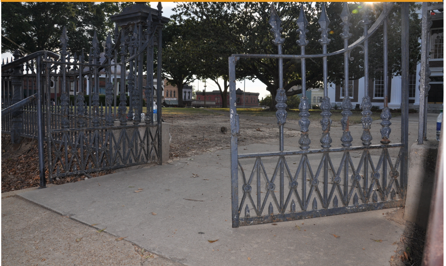
06 | Northern Fence Gate: sagging.
