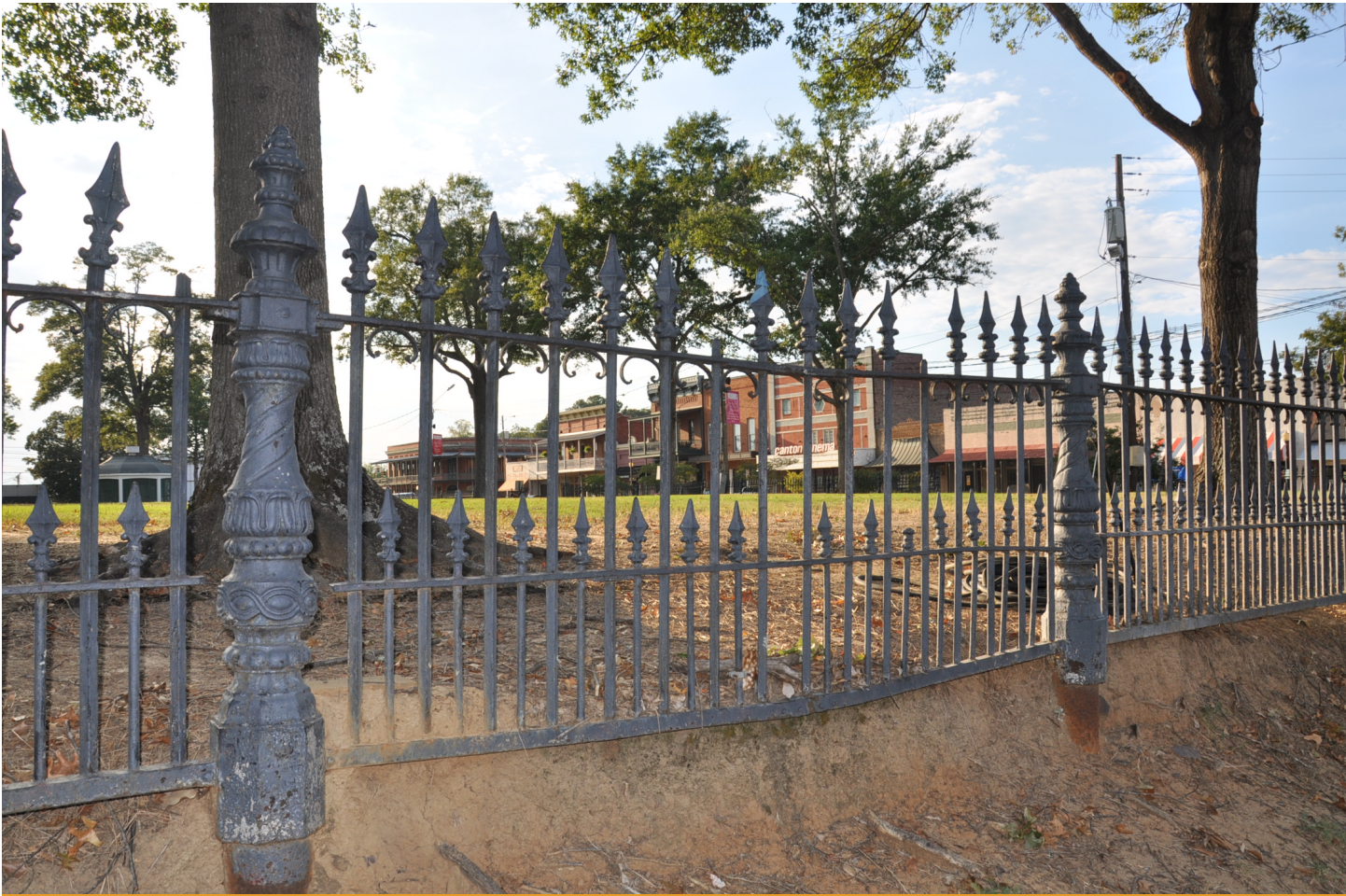
14 | East side of fence: Rusted out post bottoms and invasive roots.
