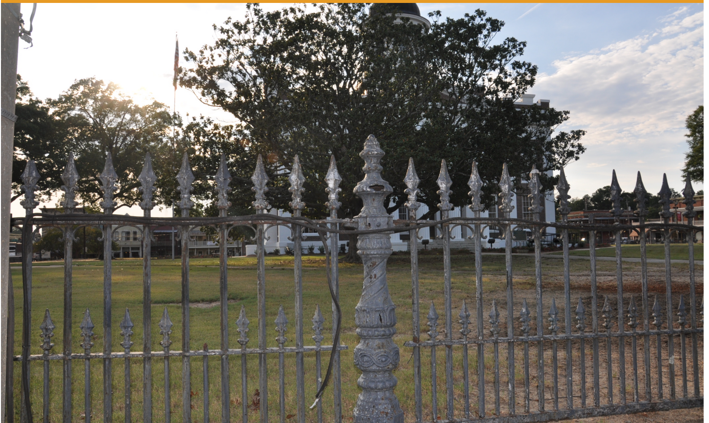
04 | East side of fence: rusted through post.
