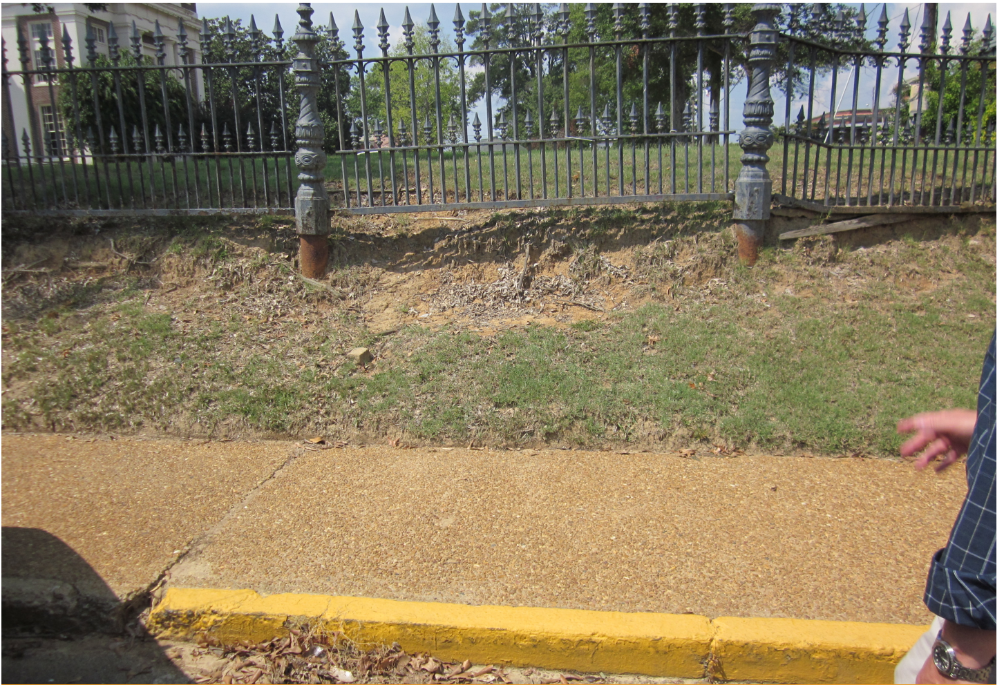
08 | East side of fence: rusted out post and sagging.
