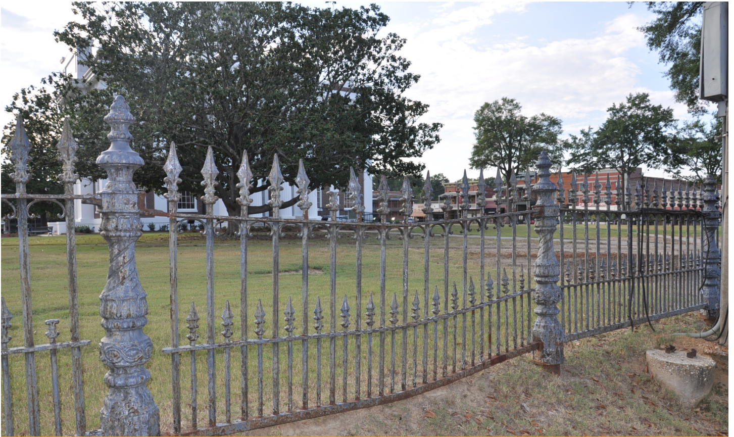
03 | East side of fence: broken finial and sagging center.
