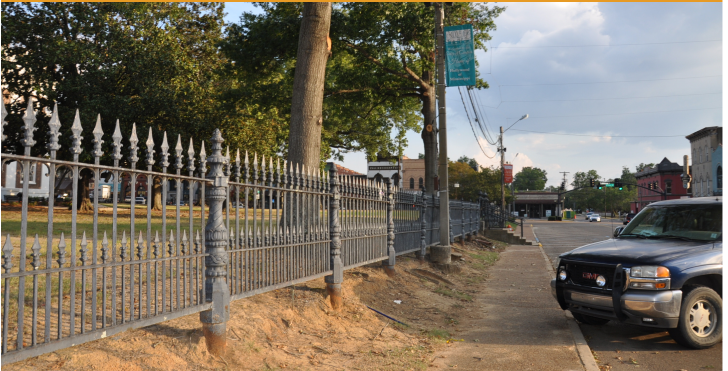
09 | West side of fence: rusted out post.
